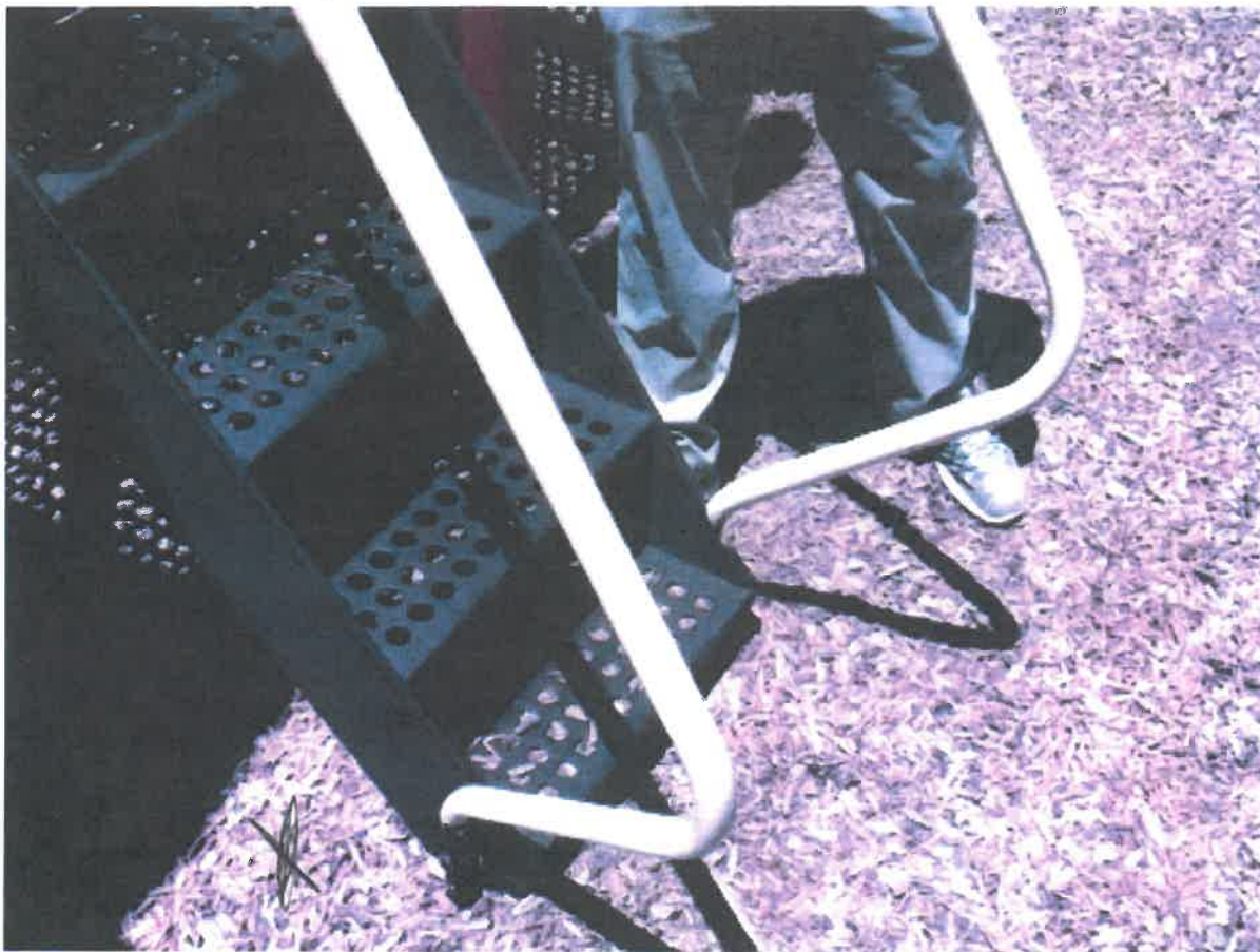
PLAYGROUND LADDER HANDRAILS ARE LOOSE AND COULD GIVE WAY.
