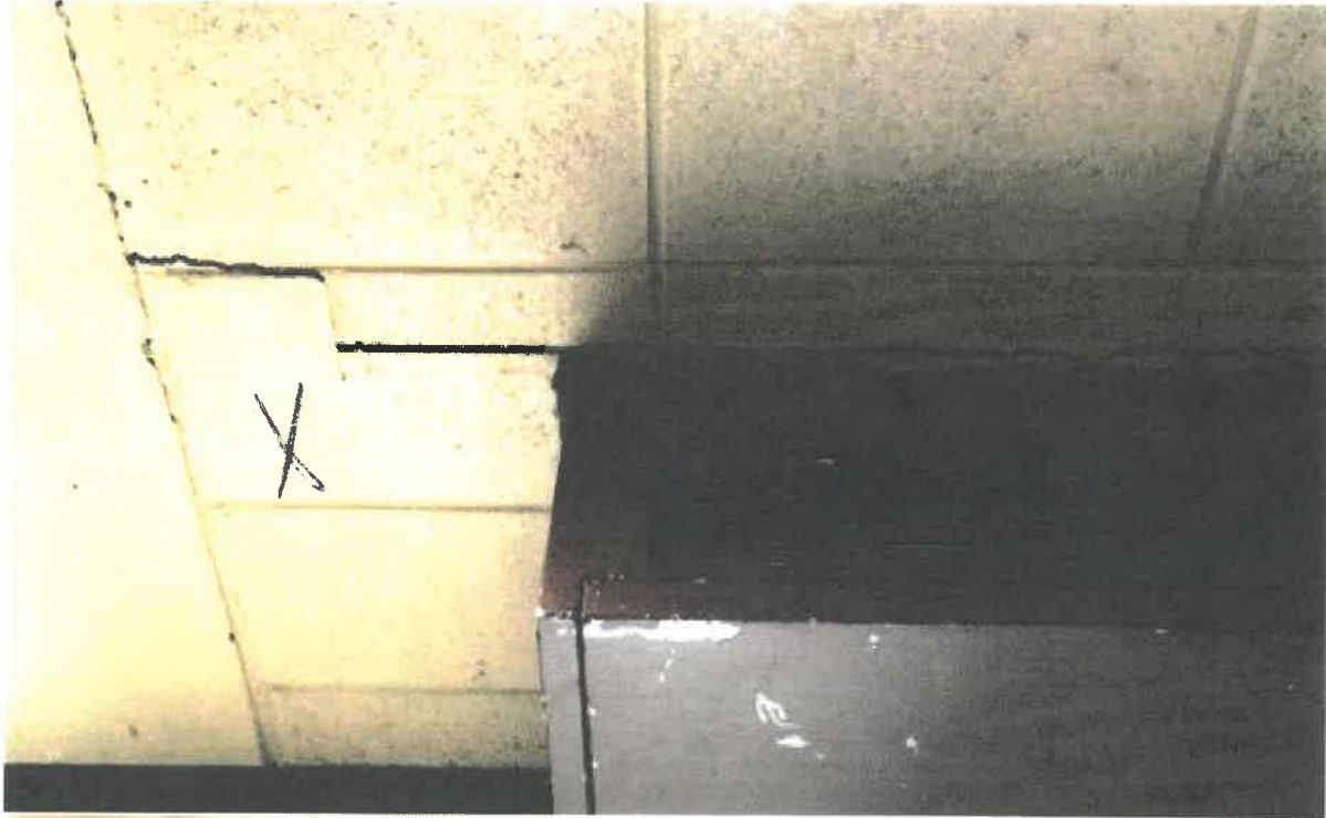
CRACKED WALL AROUND OLD WALL HEATERS.
